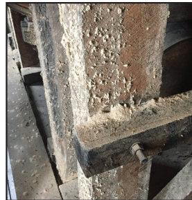
Rickhouse inspection showing heavy accumulation of frass from powderpost beetle activity.
